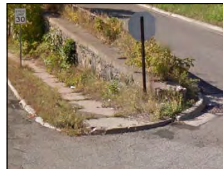
Figure 7.6 | Non-ADA compliant sidewalk at Piedmont Avenue & W 2nd Street
