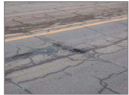
Surface cracking and pavement deterioration
